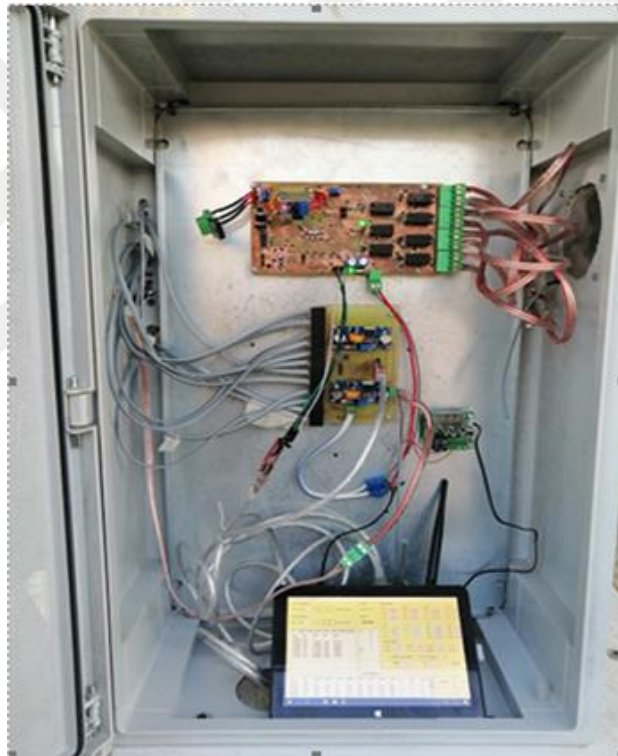
Figure 3.2 PPMAS junction box
