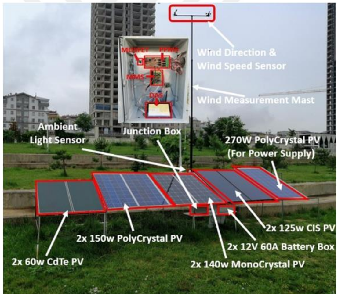
Figure 3.4 PPMAS system, pv panels, and wind measurement mast.
