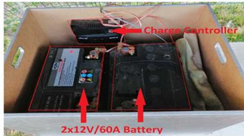
Figure 3.41 Batteries and charge controller in the power supply
