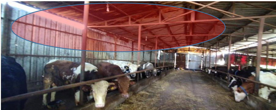
Figure 7. Example of corrosion in structural elements
